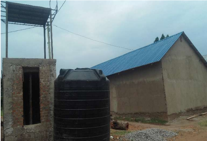
Girls' dormitory (not complete) by Dutch NGO Constructed tank stand and bought a 10,000 liter tank (not complete), by NGO from netherlands through Stichting Morkiswa
